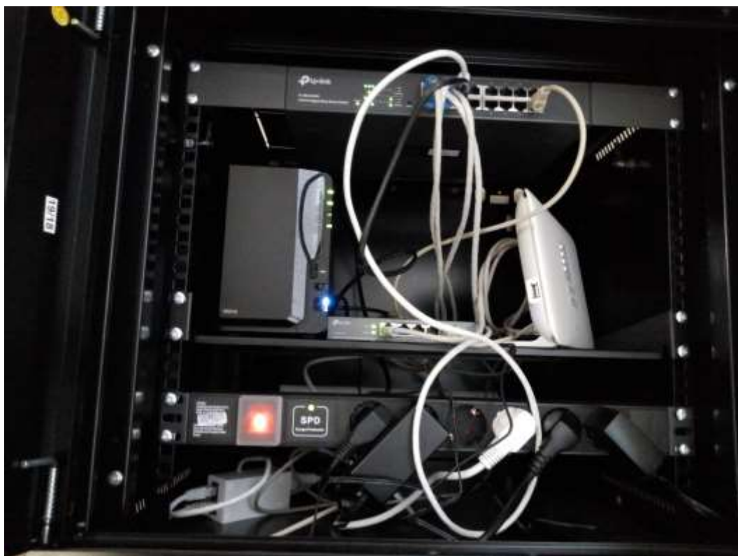
6. ábra Router, switch, NAS
